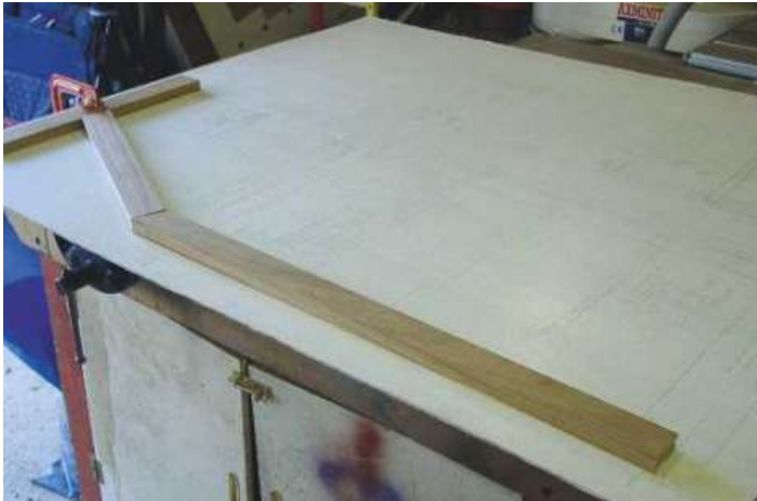
▲ Pic.1 Make a full-size drawing of the outer frame so that you can lay out the components, especially the angled joints for the flap
